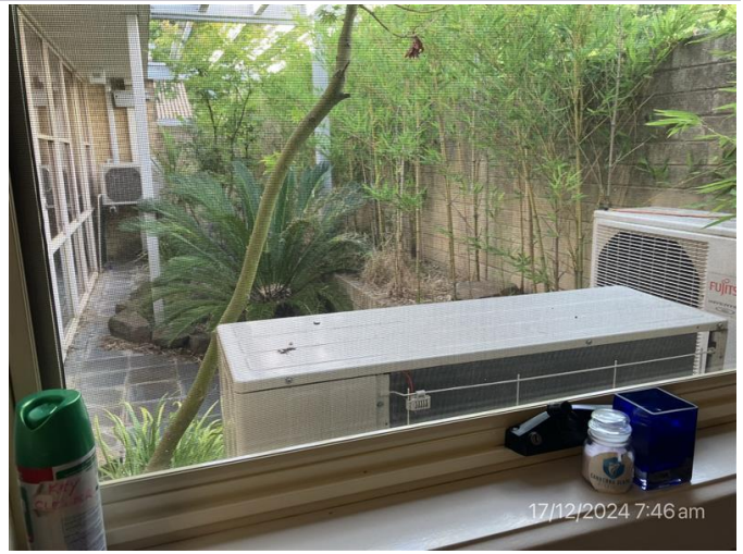
Split system air-con
