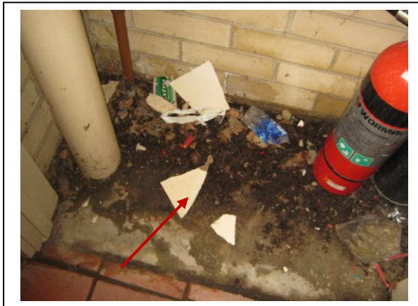
Photograph 5: Fire hose reel cupboard adjacent unit 12 – sheet debris on ground (refer sample 5864 – A5) No Asbestos Detected
