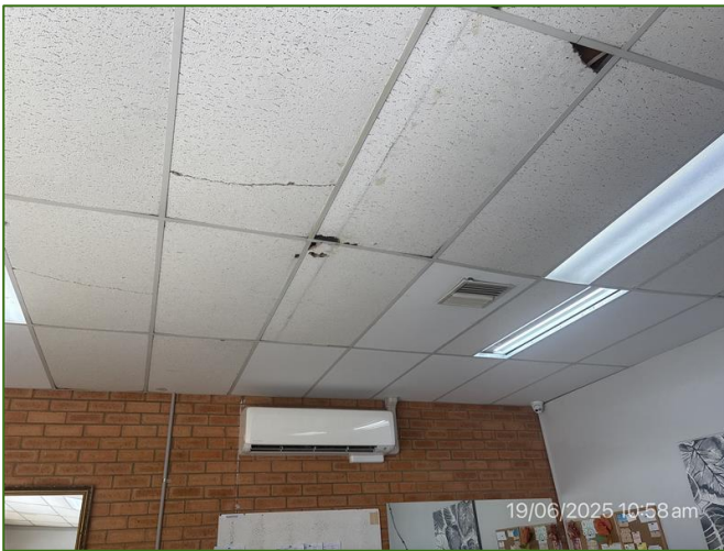
Split-system Air Conditioner
